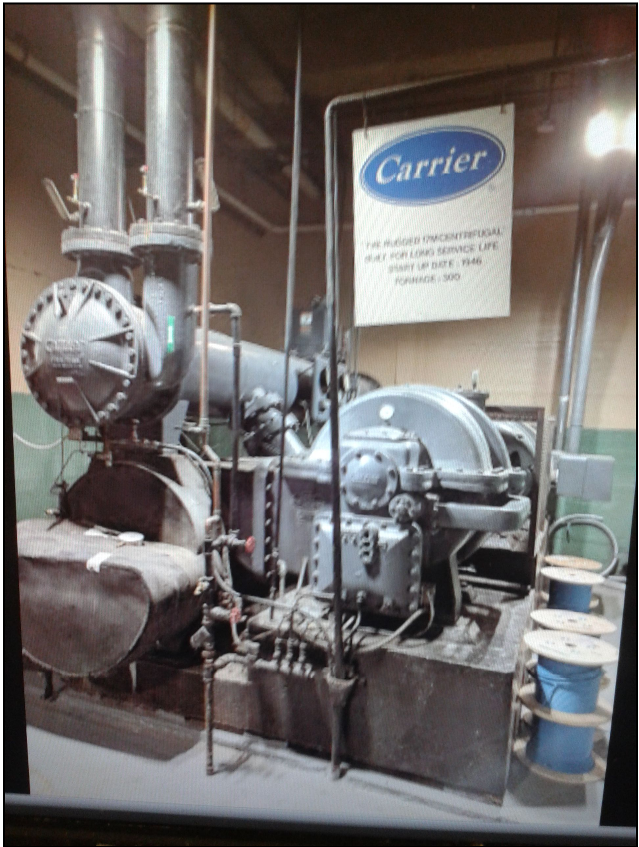
On display at the Fox Theatre in Atlanta, Georgia in 1999 The Carrier 300 TR centrifugal chiller installed in 1946 for the air conditioning
